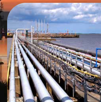
Condotte marine / Sealines
